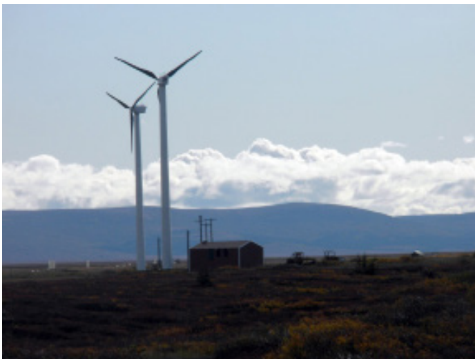
Northern Power 100B turbines, photo courtesy of AEA.
